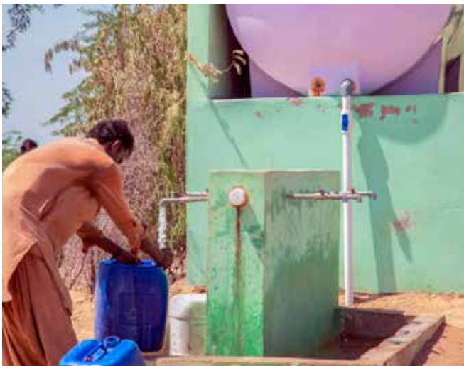
Paylaai from Satla Bheel village Pakistan fills water from the newly installed water plant using a solar pump. Photo: Concern Worldwide 2017
